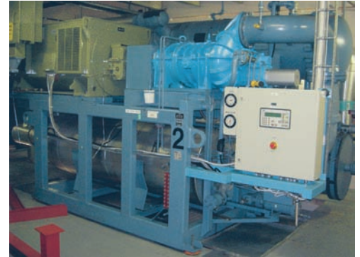
One of two heat pump units.
