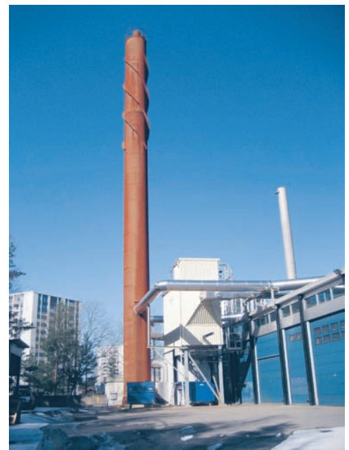
An electrostatic filter has been installed to clean the flue gas from the wood powder boiler.
