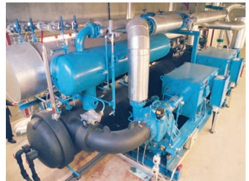
One of three chillers now installed
