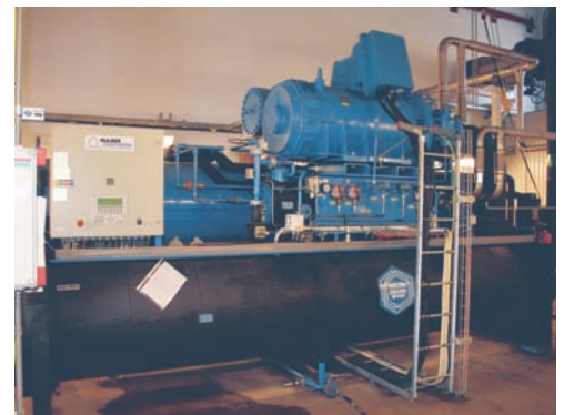
One of three chillers now installed
